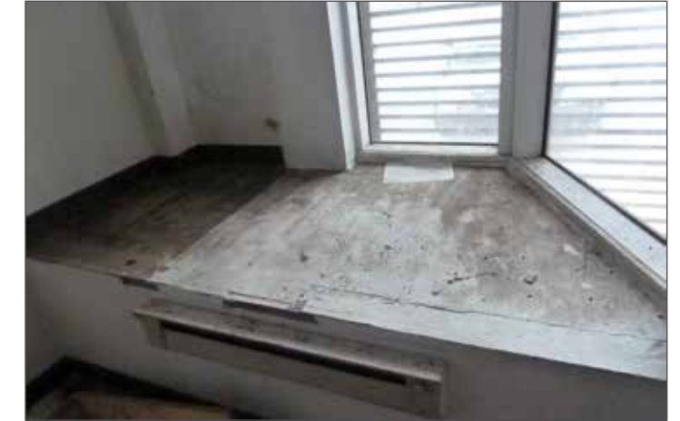
The existing storefront windows are intact and should be preserved for future use. The window glass need to be replaced and the bay area need some repair.
