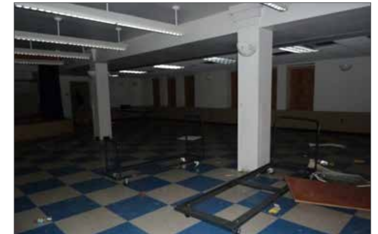
Community room on second floor (on east side of building) shows concrete frame structure in good condition; the floor finished need to be changed and the exterior windows need to be replaced complimenting historic character of the building
