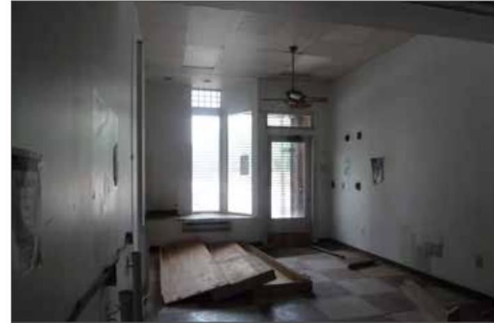
The central bay on first floor was occupied by a laundromat; the building needs major clean-up from inside by removing the debris.
