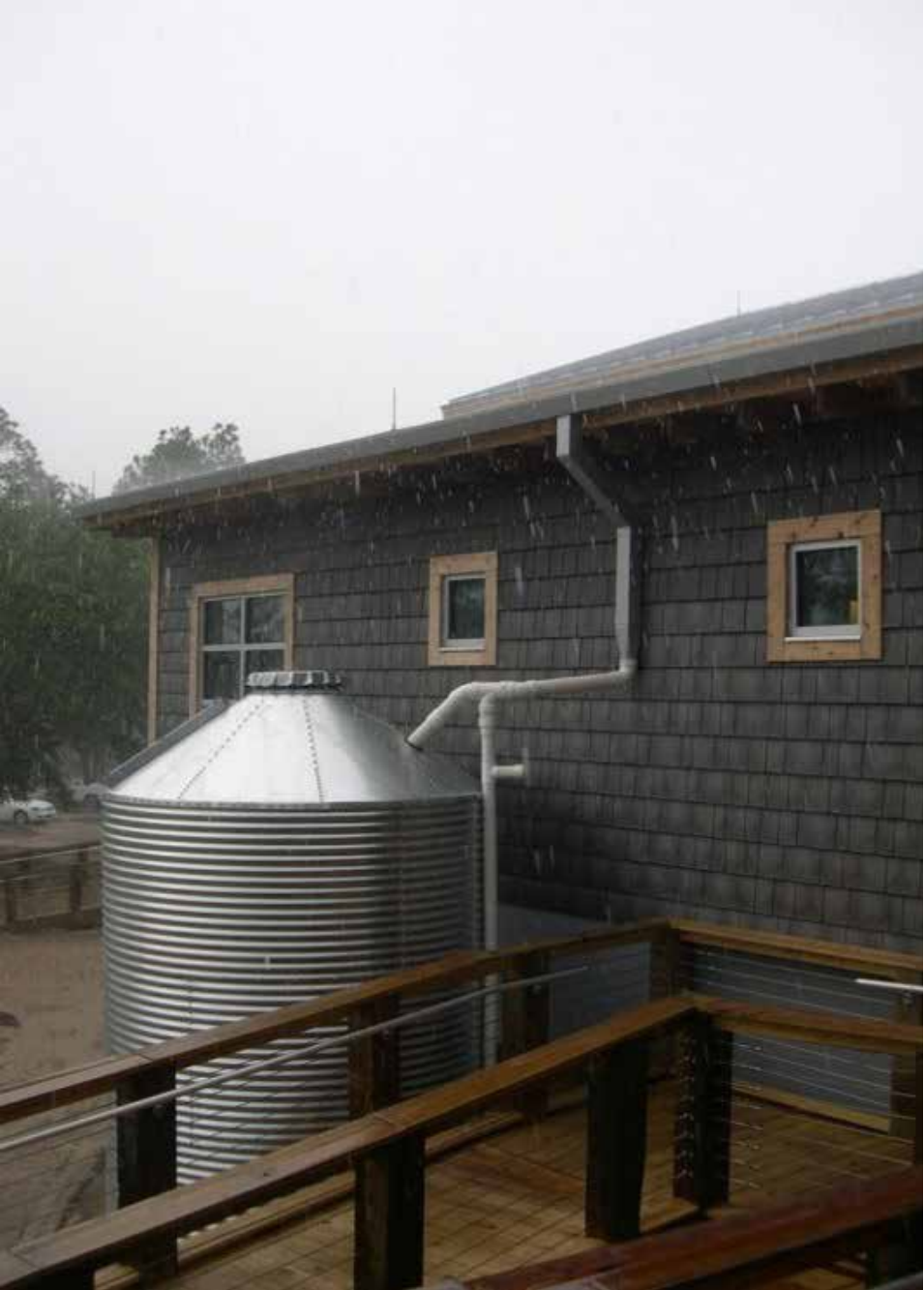
Harvesting rainwater to irrigate the gardens captures a resource that normally goes down the drain, reducing the building's reliance on costly city water
