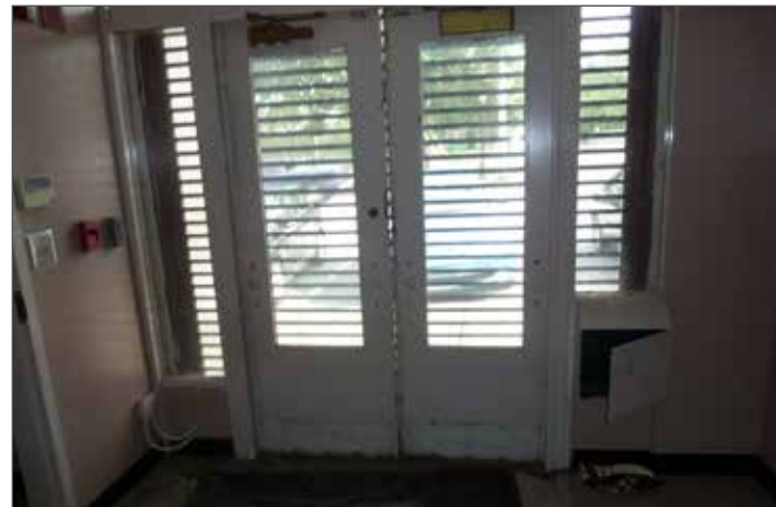
Main door on first floor providing ADA access from Atlanta Student Movement Boulevard; it could be preserved with minor repair.
