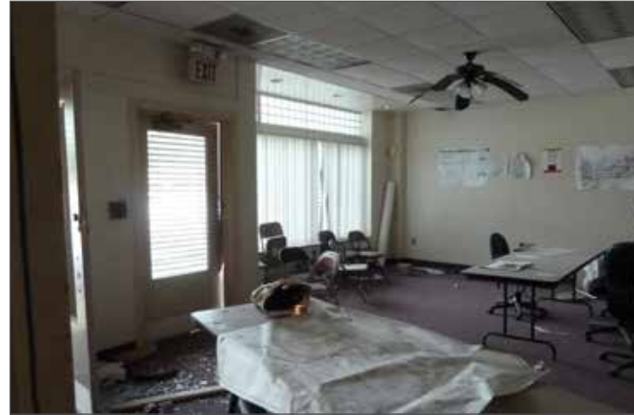
The building interior is in distressed condition; including the partition walls, ceiling and carpet. The old furniture and fixtures need to be removed.
