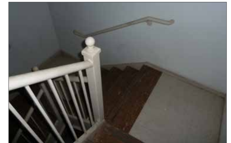
Egress stair on west side of second floor; the stair provides fire exist and should be preserved
