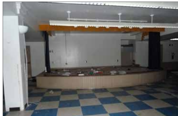
Existing stage in the community room; it could be repurpose or removed based on the future program needs in the building
