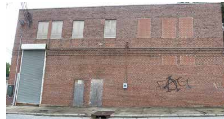
E. West elevation on Roach Street, boarded up/filled doors and windows
