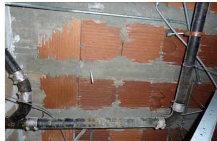
Building slab made of clay tiles and concrete; the structural condition should be examined by a structural engineer for stability and water proofing
